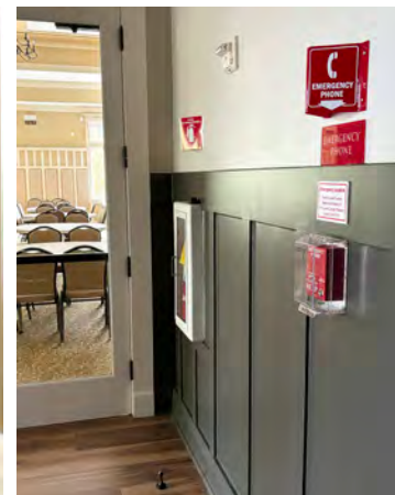
▲ An emergency phone that connects directly to Emergency Responders is located right outside the Ballroom door, along with a fire extinguisher.
